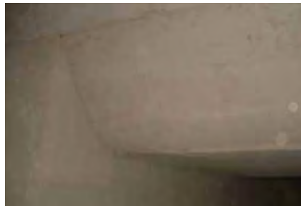
Riser duct lined with 56l Denscast SIC 30
