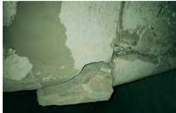
Damage area caused by chemical attack and insufficient expansion.
